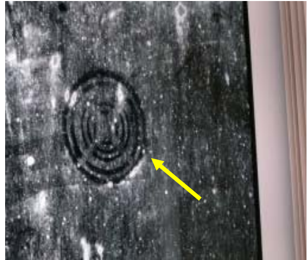
Photo Above shows an installed window with heavy condensation on Glass. Different patterns are visible within the condensation including the outline of a Vacuum Cup mark which may have been used to handle the glass during fabrication or installation. There are no visible marks present on this glass in the absence of condensation.
