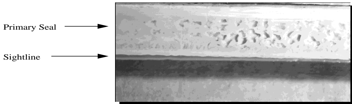
Gas entrapment in primary seal due to pumping of the seal during weather cycling (low modulus secondary seal)
